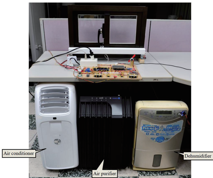
Fig. 15. (Color online) Smart home environment control system in operation.
