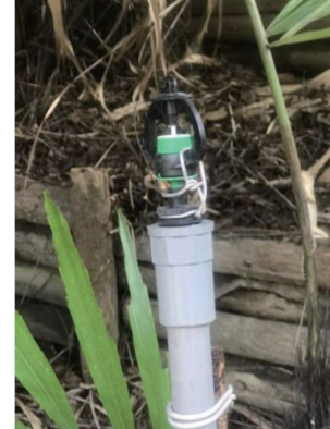
Fig. 20. (Color online) Sprinkler head.
