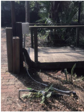
Fig. 18. (Color online) Connection of controller and water pipe.
