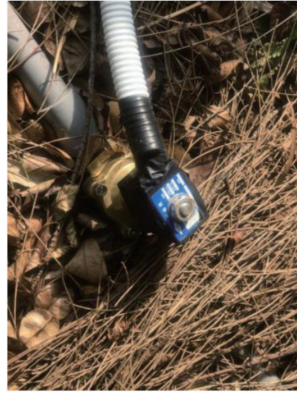
Fig. 19. (Color online) Connection of solenoid valve and water pipe.
