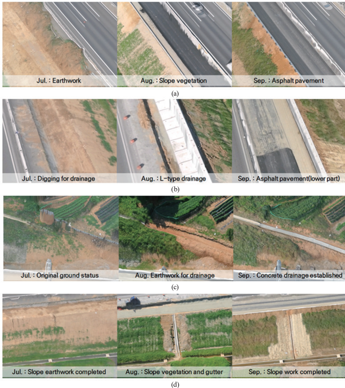
Fig. 5. (Color online) Change monitoring of (a) earthwork and asphalt pavement, (b) drainage work at the road, (c) drainage work at the mountain, and (d) slope work at Pyeongtaek–Seopyeongtaek expressway construction site.
