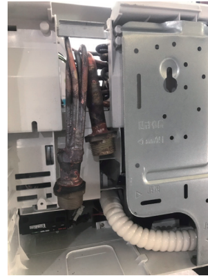
Fig. 4. (Color online) Indoor evaporator unit water distributor pipe.
