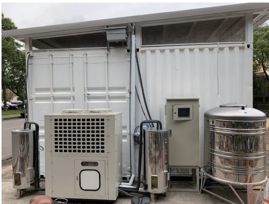
Fig. 5. (Color online) Heat pump and heat recovery system.
