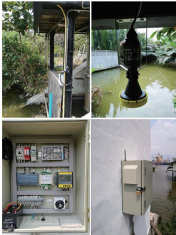
Fig. 8. (Color online) Example of measurement installation.
