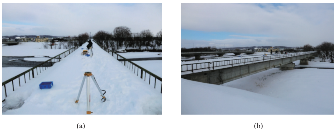
Fig. 10. (Color online) General view of Mukagawa Bridge in winter. (a) Front view and (b) side view of the bridge.
