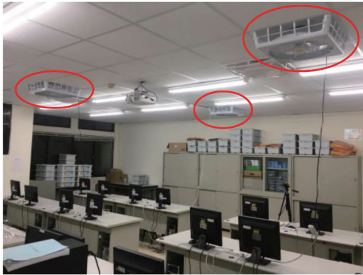
Fig. 9. (Color online) Fan installation location.
