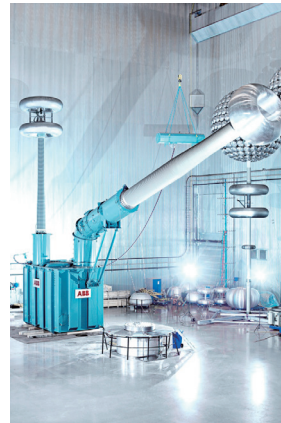
Fig. 2. (Color online) Converter transformer at \pm 1100 kV.
